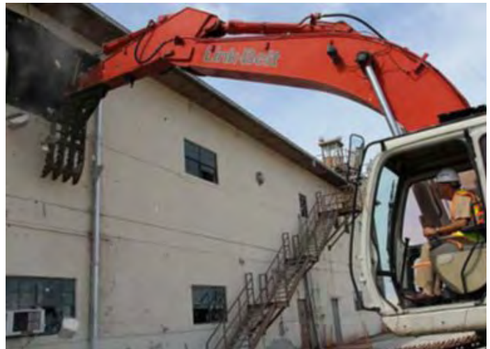
NAS Jax CO, CAPT Howard Wanamaker, uses an excavator to tear down part of Hangar 113, following a ceremony Aug. 24. Additionally, Hangars 114, and 115 are also being torn down due to the age and non-use of the facilities.
